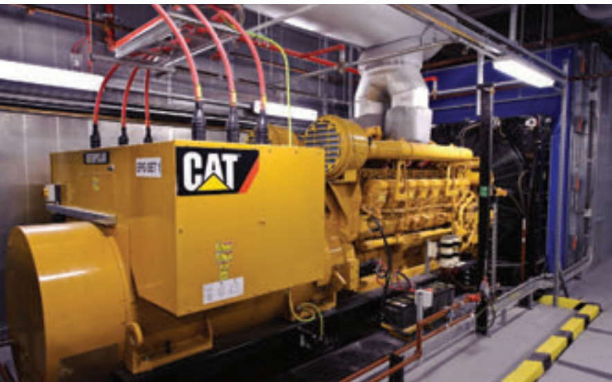
Above and right: The tri-generation system comprises a combined heat and power engine linked to an absorption chiller. Facing page: Active chilled beams are driven by air from the ventilation system.
