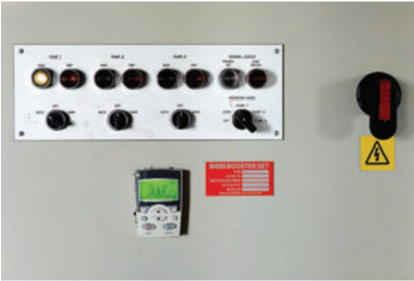
Top: The chiller system. Bottom: Variable speed pump control panel.
