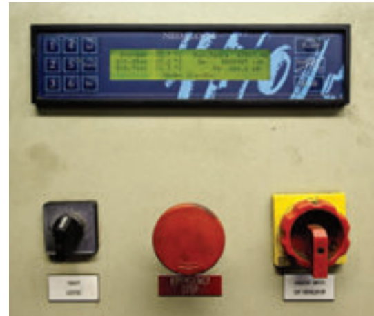
The combined heat and power unit links to three gas boilers.
