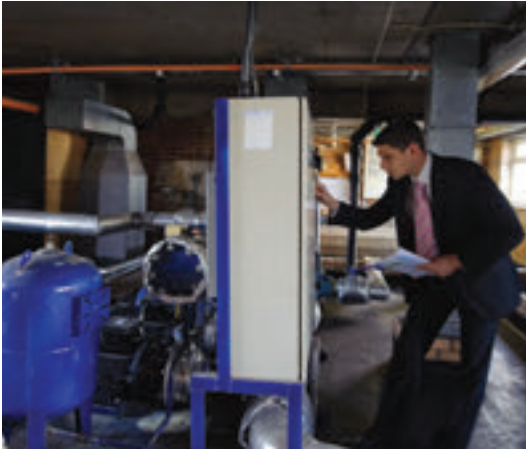
Alexandros Balaskas checks the combined heat and power unit.
