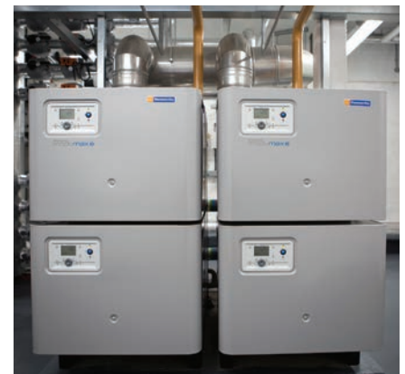
Figure 6: Four 254kW modular gas condensing boiler sections that combine to provide the heating for St Paul's Cathedral
