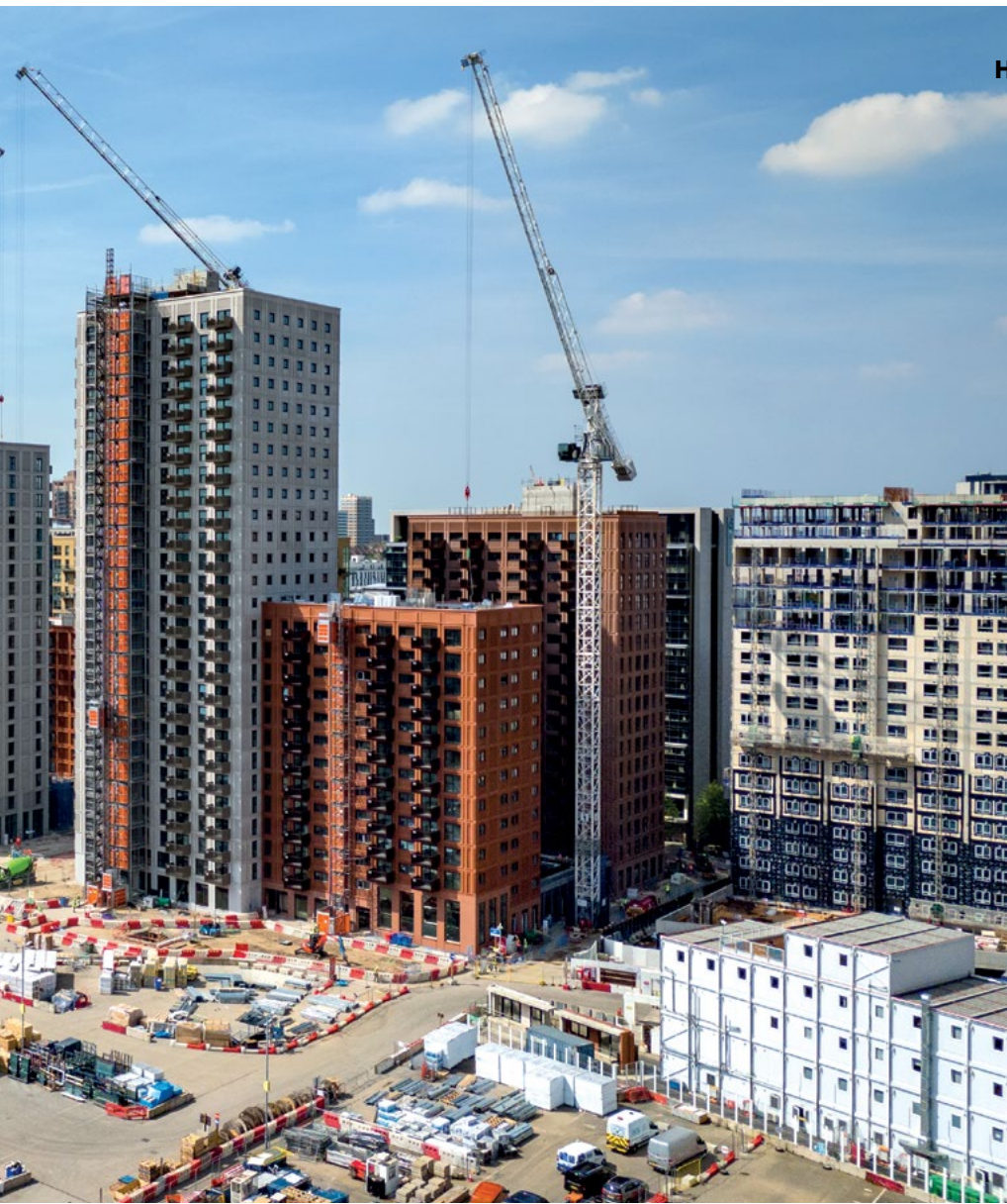
The site welfare facilities for the Wembley Park residential project are in the bottom right-hand corner
