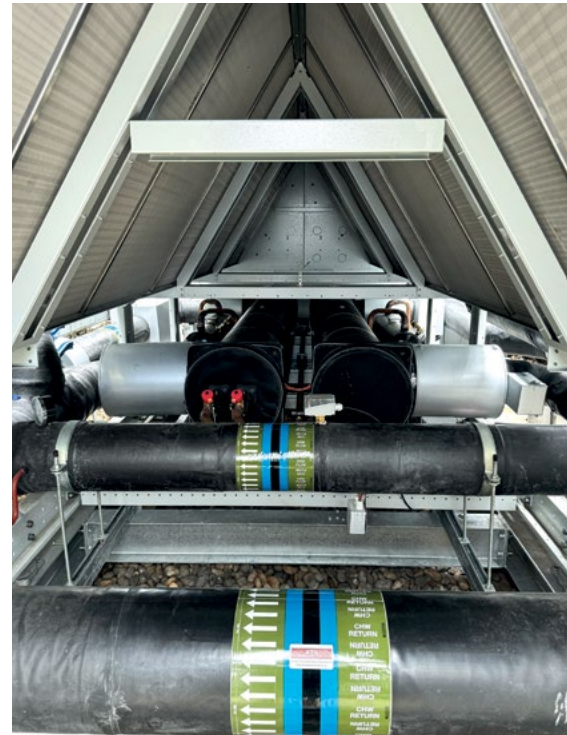
Inside a 4-pipe simultaneous heat pump
